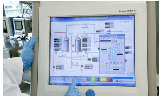
The HMI of the control system as interface between the process and the operator
